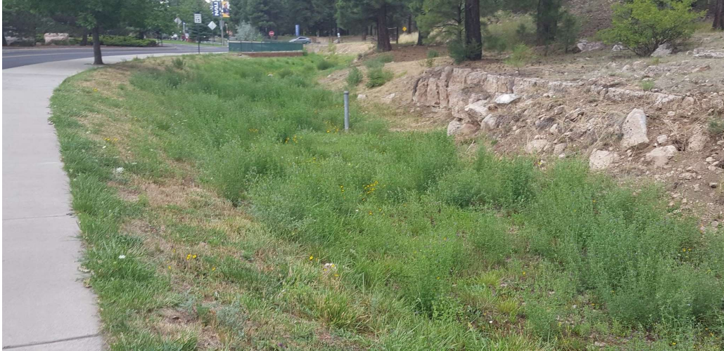
Figure 1.3 - Overgrown vegetation in portion of Sinclair Wash
